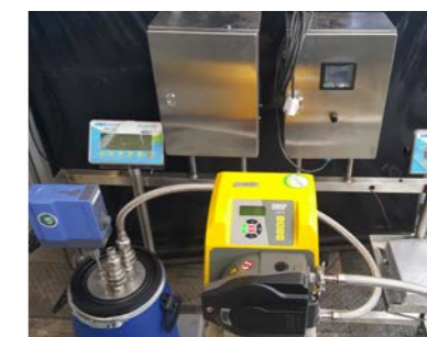
Rotary drum filtration unit
